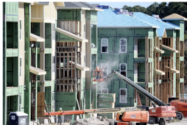
Workers finish the exterior of new apartments under construction in Clearwater, Fla., Dec. 28, 2022.
